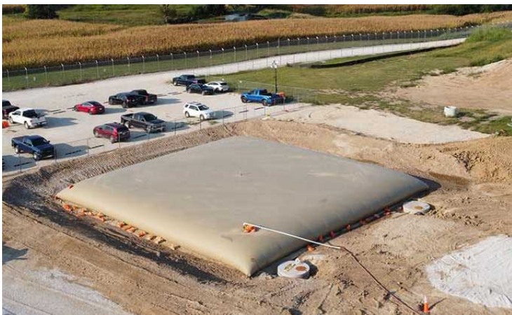
Emergency Potable Drinking Water Storage Tanks and Bladders
